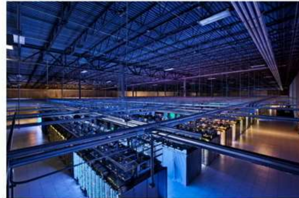
Google's data center, Council Bluffs, IA https://www.google.com/about/datacenters/gallery
